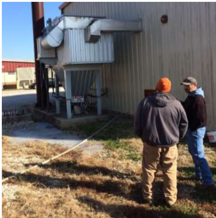
The emissions system installed in Steelville captures solids and ash from the smoke.
