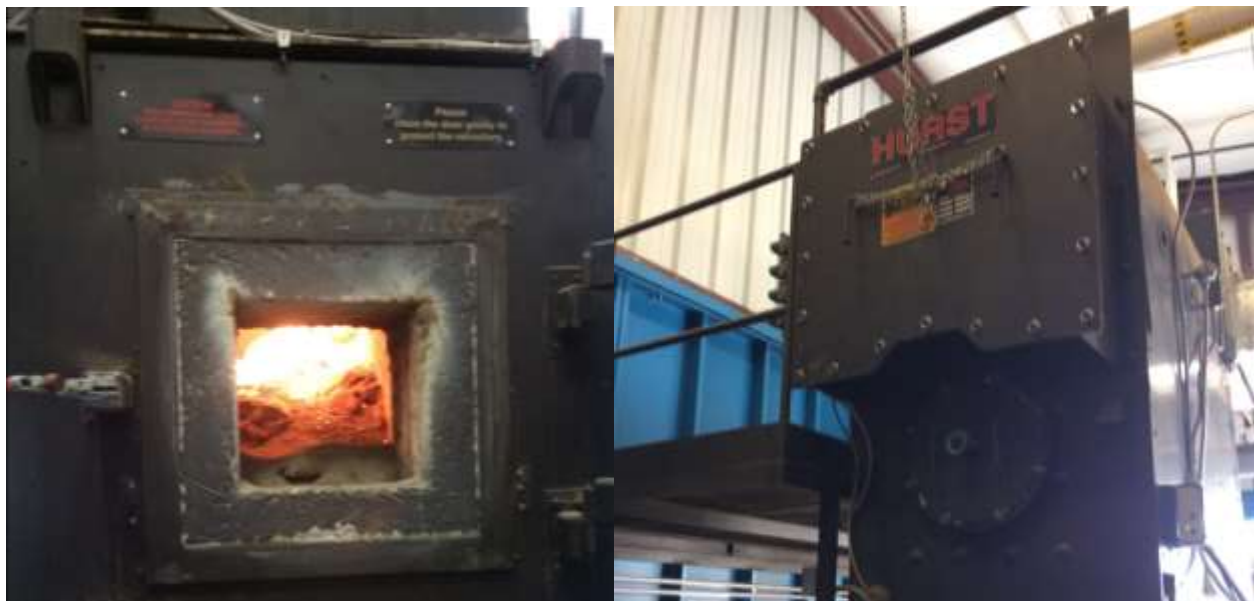
Left: The computer-controlled system requires minimal maintenance as the wood chips are fed in to the furnace according to heating demand. Right: The boiler heats fluid stored in a large tank, which transfers this heat via a closed-loop system of tubing, and is circulated to heat exchangers throughout the school buildings.
